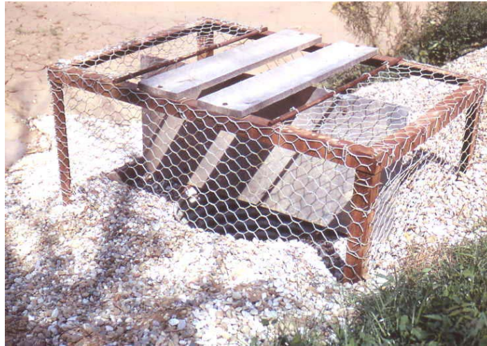
Figure 2. Drop inlet pipe with anti-vortex baffle and trash rack
