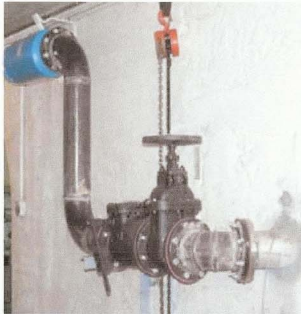
The air intake system and valves for the draft tube aeration system at the 18-MW Lloyd Shoals plant take air from the upstream bearing gallery and feed it to the draft tubes to increase dissolved oxygen in the water.
