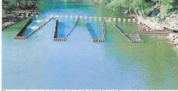
The aerating weir installed at 18-MW Lloyd Shoals in 1991 increased downstream dissolved oxygen (DO). However, a 1994 flood damaged the weir and significantly reduced its effectiveness. Because the new draft tube aeration system installed at the plant raises DO levels to sufficient levels, Georgia Power removed the weir.
